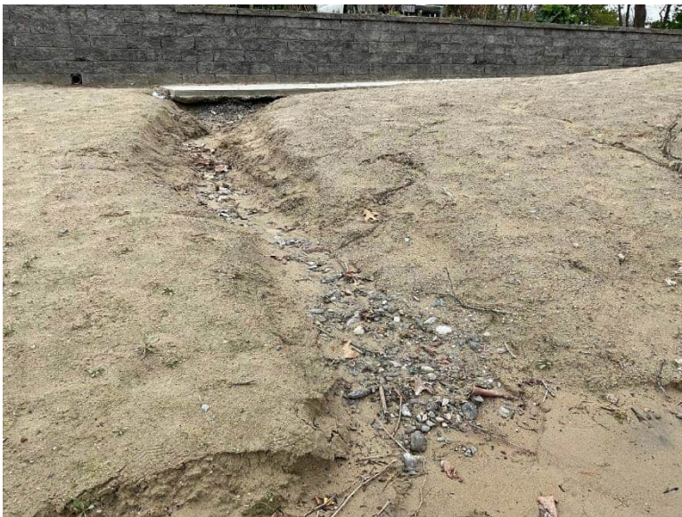
Significant erosion from sidewalk to bank is causing undercutting of concrete.
